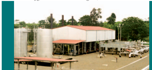
Petroecuador, 3 x Cat® 3612 crude fuel pumping packages, Ecuador
