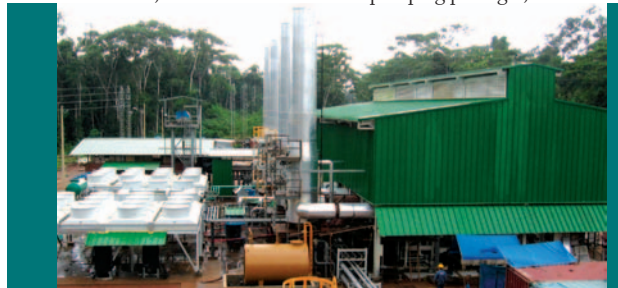
Pluspetrol & Ferrenergy, 4 x 16PA6B heavy fuel gen sets, Peru
